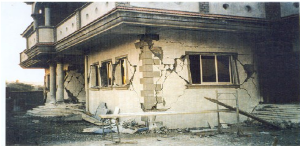
Large windows openings close to corners and short column failures
