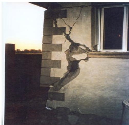
Diagonal cracking at corner column caused by twisting of frame and short column failure
